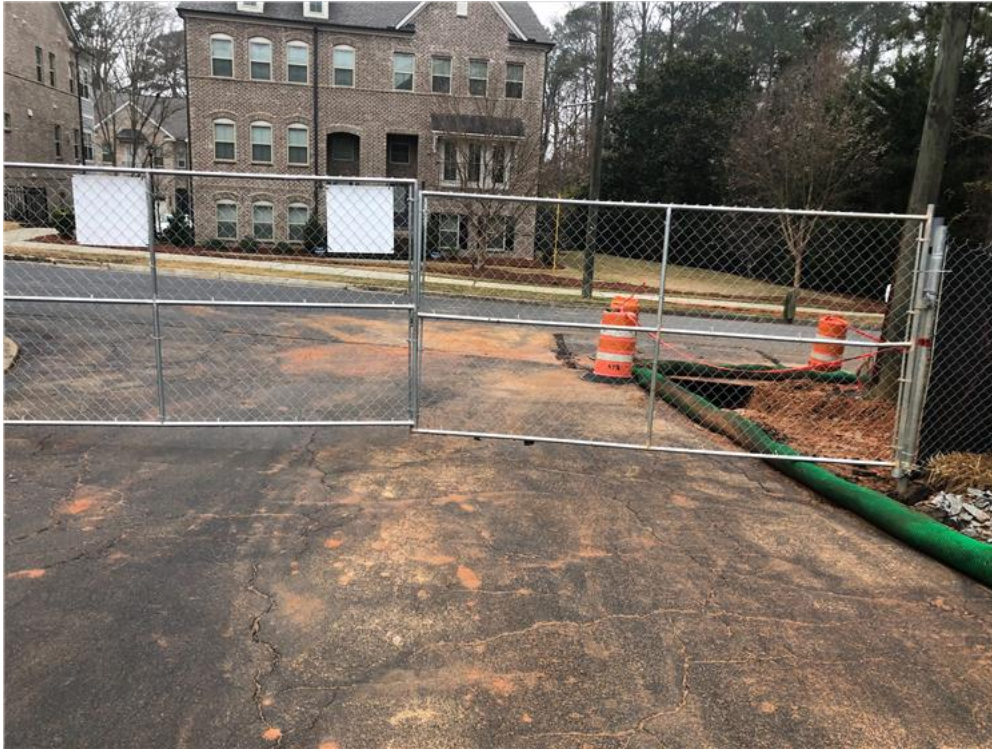
Sediment tracking onto public right-of way
