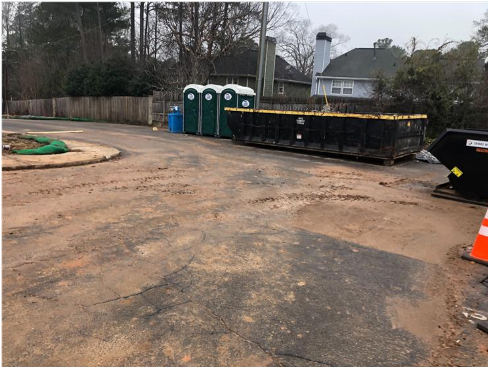
Sediment tracking onto the parking lot
