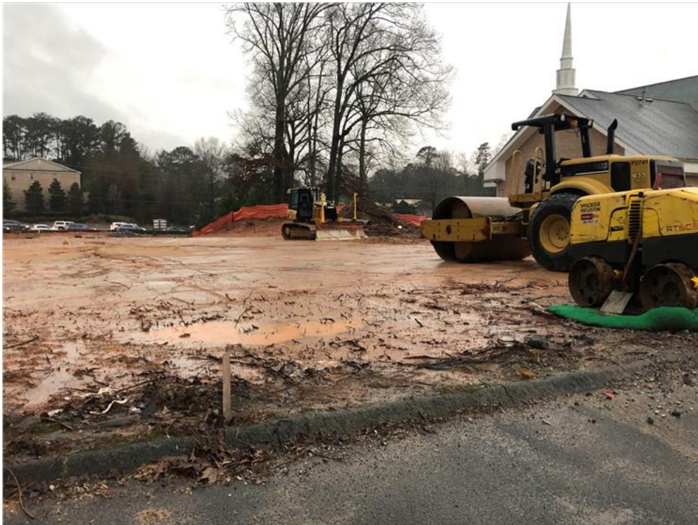
Sediment trap ( needs a sediment trap to keep soil from going into public street)
