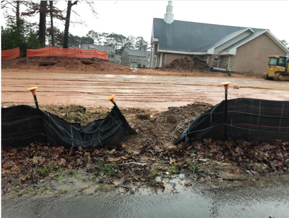
Silt fence ( maintenance is need to keep soil from going into public street)
